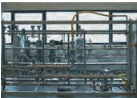
BOLL & KIRCH gas test-bench
